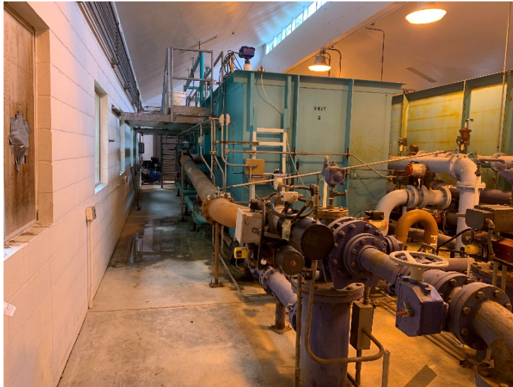
Figure 6 – Filter #2, Currently Inoperable
