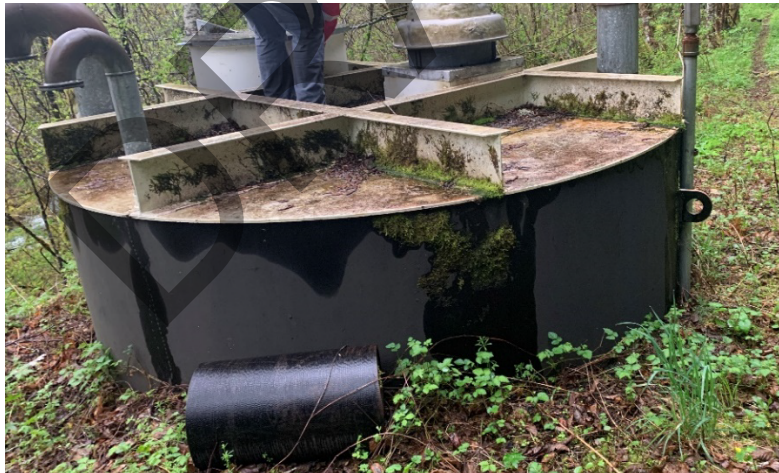
Figure 4 – Alder Creek Raw Water Pump Station
