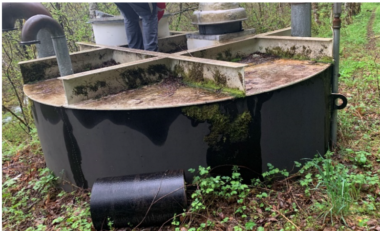
Figure 4 – Alder Creek Raw Water Pump Station
