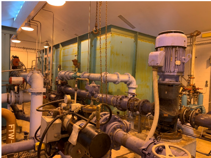
Figure 7 – Filter #3 and Single Finished Water Pump
