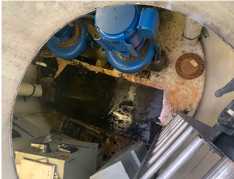
Figure 5 – Looking Down Into the Alder Creek Raw Water Pump Station
