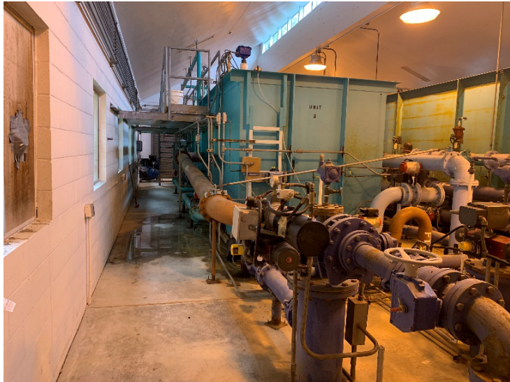
Figure 6 – Filter #2, Currently Inoperable
