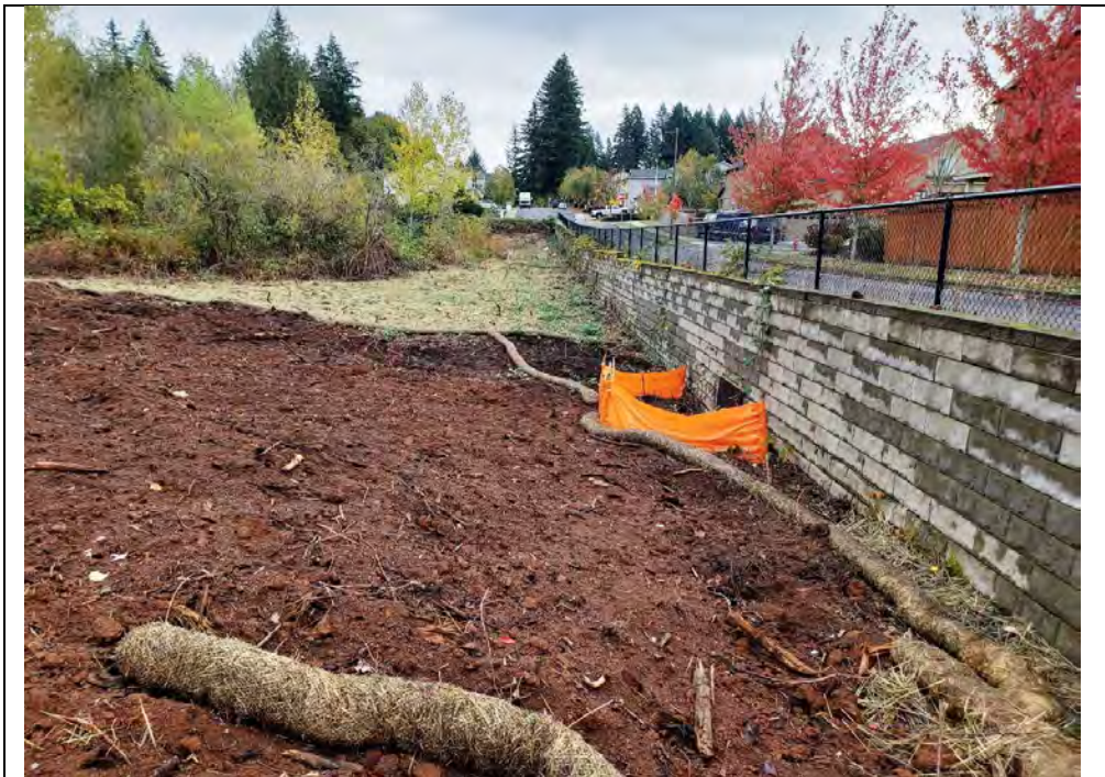
Photo 8 Track "E" after Blackberry clearing along Olson Road in preparation for the road widening. Photo looks East toward Jewelberry Road. ETC Photo 10/30/2018.
