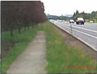
Sidewalk Below Grade
