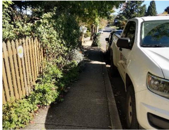
Encroaching vegetation along sidewalk on north side of Pleasant St east of Smith Ave.
