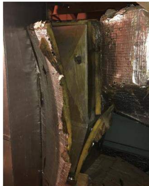
Figure M4: Damaged Ductwork Insulation
