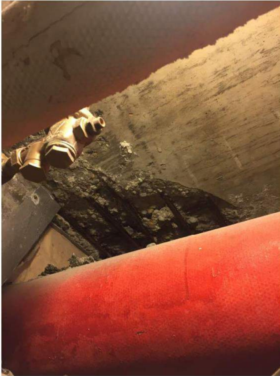
Photo 5: Corrosion of slab within pool equipment room.
