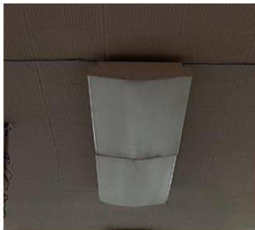
Figure E8: Typical Classroom Luminaire
