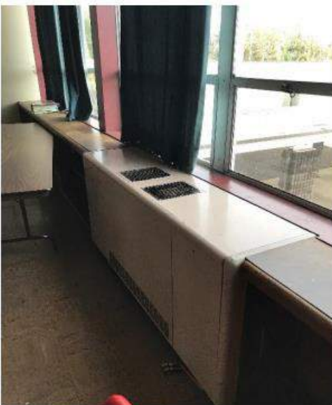
Figure M9: Unit Ventilator
