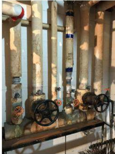
Figure P2: Cold Water Header
