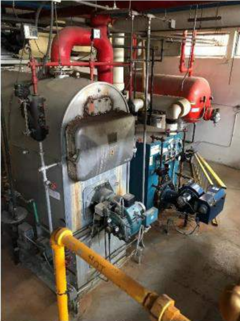
Figure M7: Original Steam Boiler
