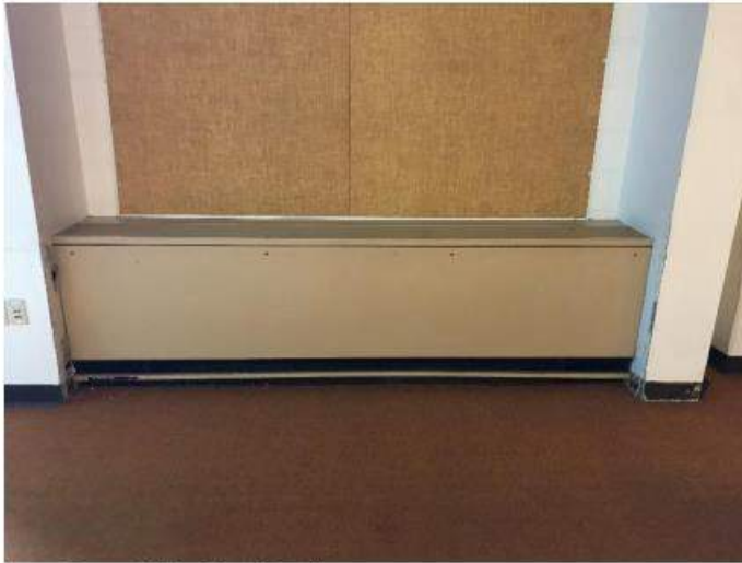
Figure M13: Unit Ventilator
