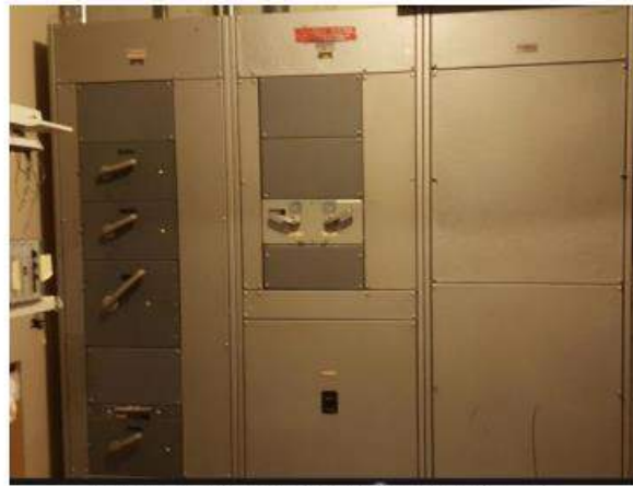
Figure E7: Main Distribution Switchboard
