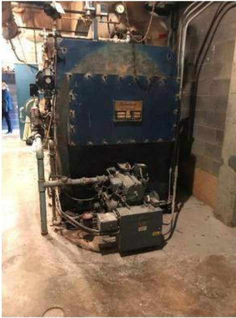
Figure M1: Steam Boiler
