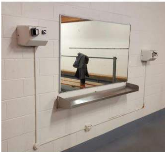
Figure E3: Surface mounted raceway
