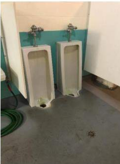
Figure P4: Floor Mounted Urinals
