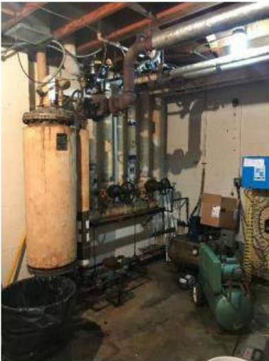
Figure P1: Hot Water Converter
