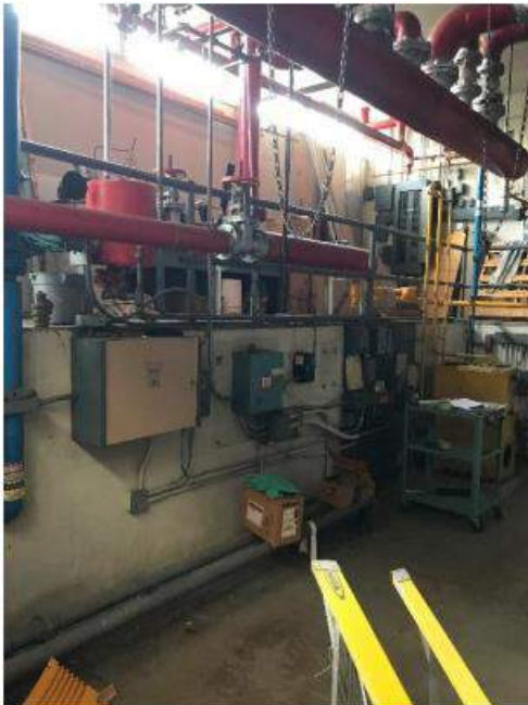
Figure M11: Boiler Room Controls
