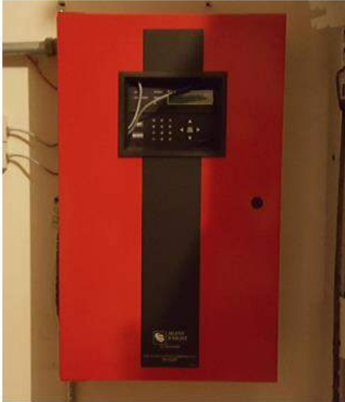
Figure E12: Fire Alarm Control Panel
