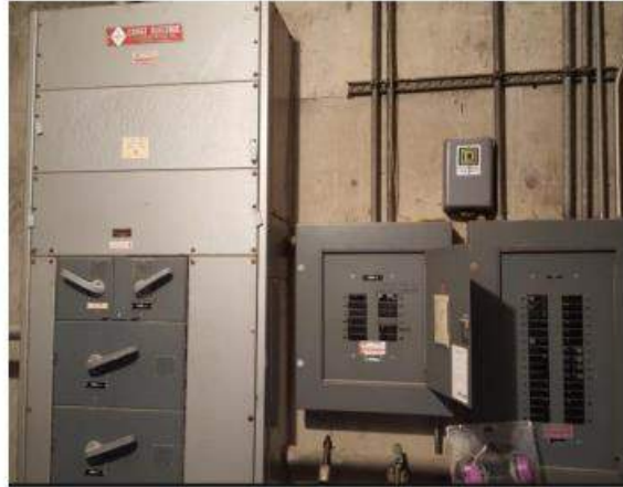
Figure E2: Main Electrical Service
