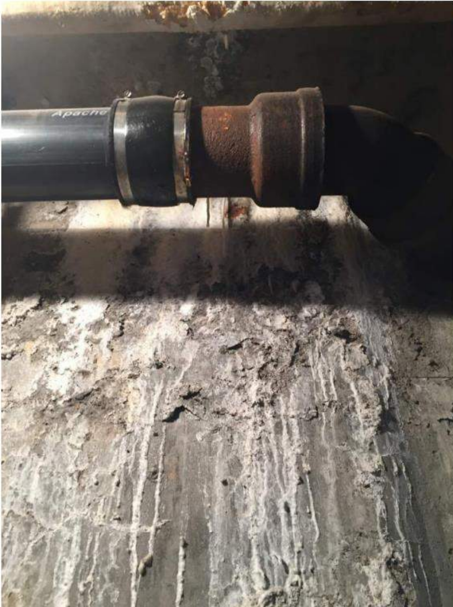
Photo 4: Corrosion along basement wall around pool perimeter.
