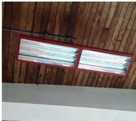
Figure E4: Pool Area Luminaires
