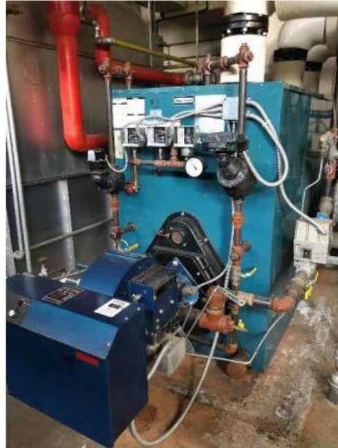
Figure M8: Newer Steam Boiler
