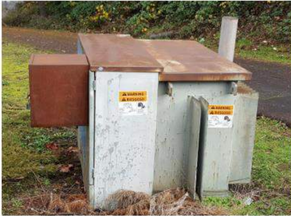
Figure E6: Existing Padmount Transformer
