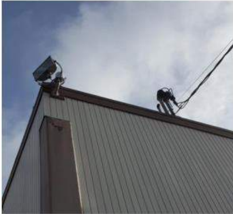
Figure E1: Utility Overhead Feed
