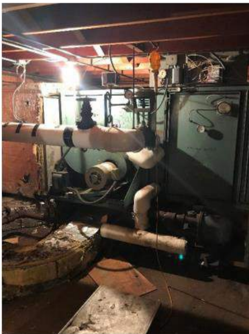
Figure M3: Air Handler and Controls
