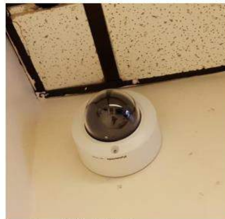
Figure E19: CCTV Camera
