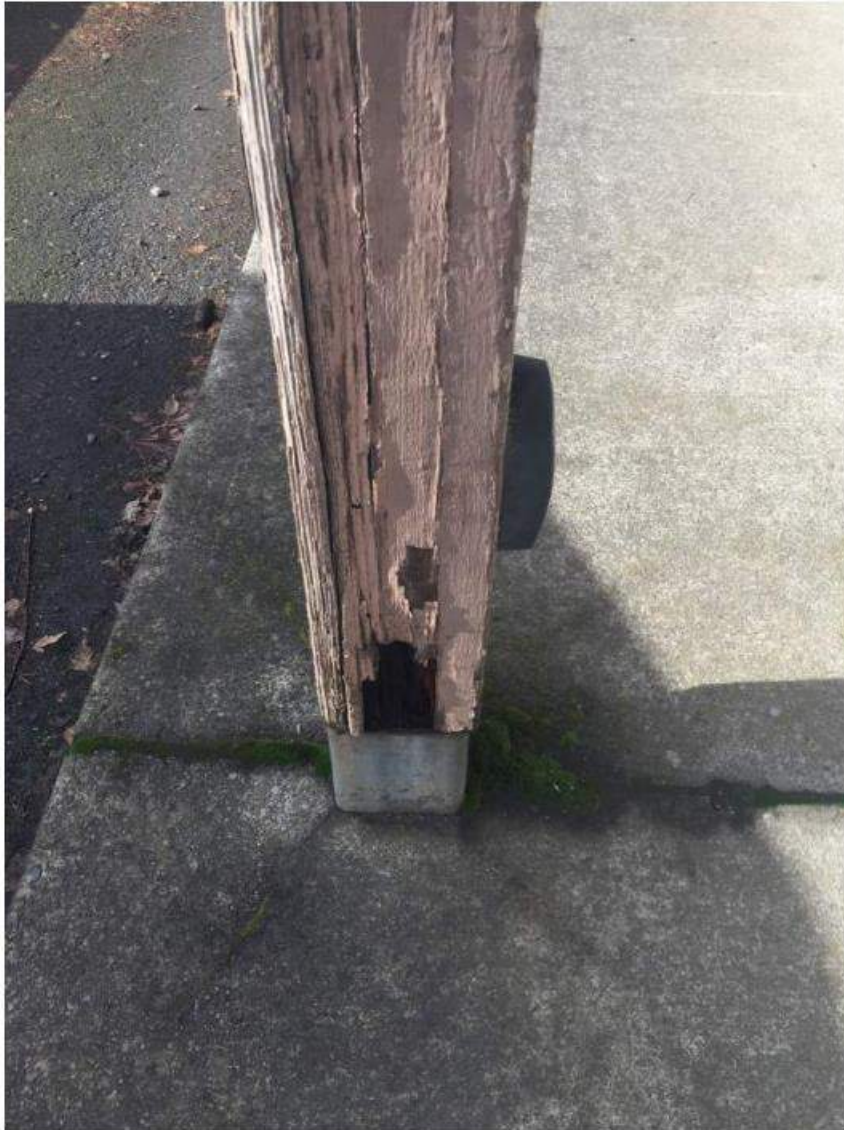
Photo 2: Deterioration at Aquatic Center entry cover posts.
