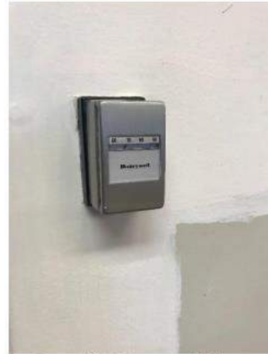
Figure M14: Pneumatic T-Stat
