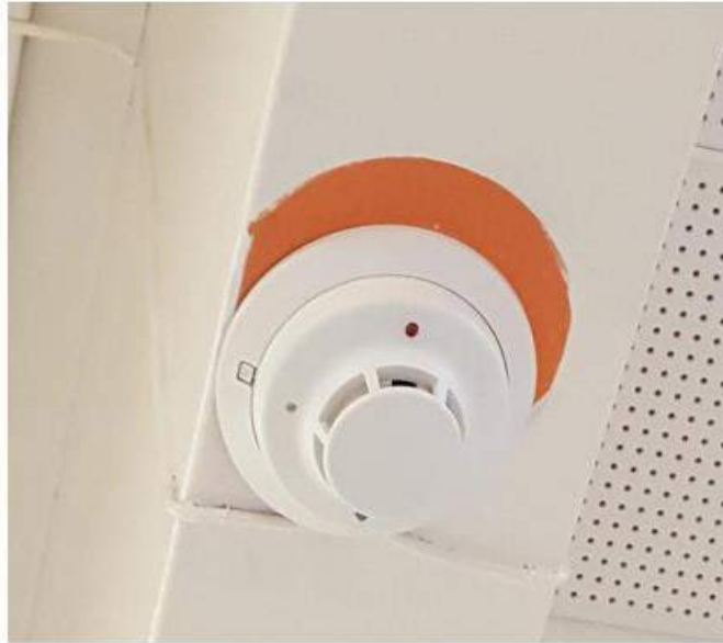
Figure E13: Typical Smoke Detector
