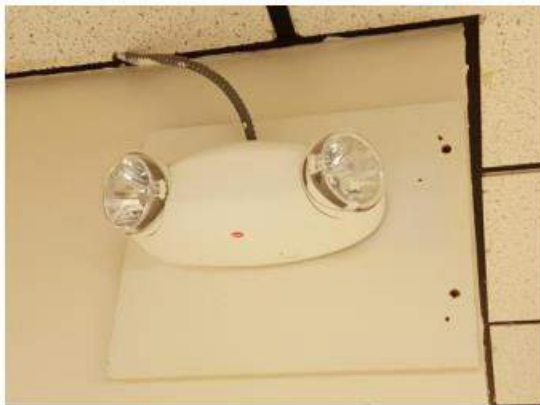
Figure E16: Emergency Wall-Pack
