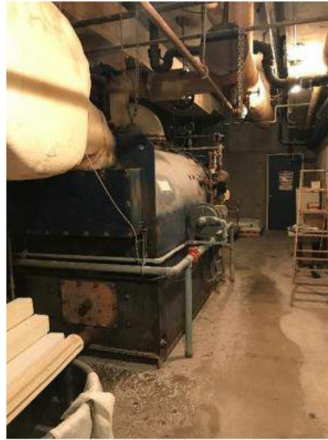
Figure M2: Boiler Room and Piping
