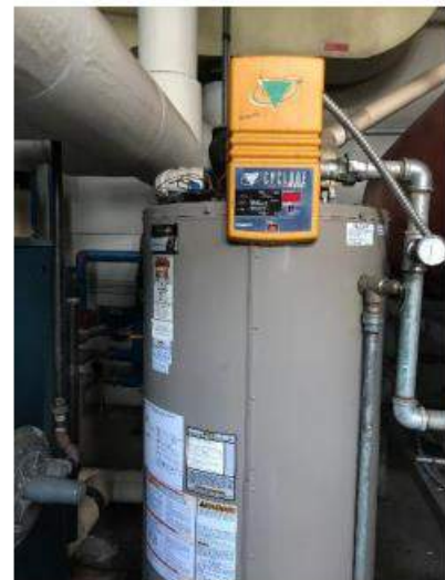
Figure P9: New Water Heater
