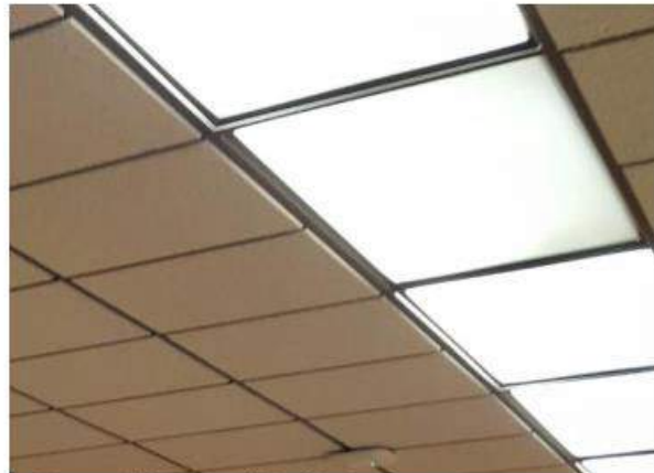
Figure E15: Typical Troffer Luminaires
