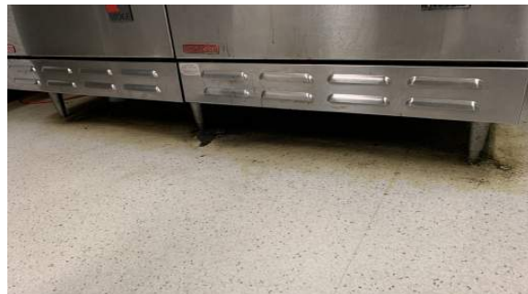
Linoleum flooring in the kitchen is beyond its life cycle and should be replaced.
