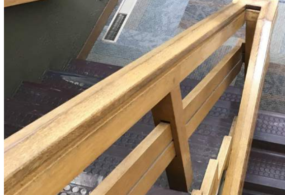
The wooden handrail is not in compliance with current code for handrail height, or width of the grip.
