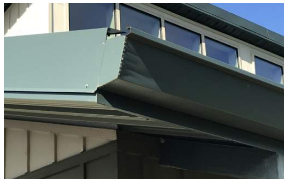
Several areas of gutter, such as this one, are in need of repair. Mechanical fasteners should not be used.
