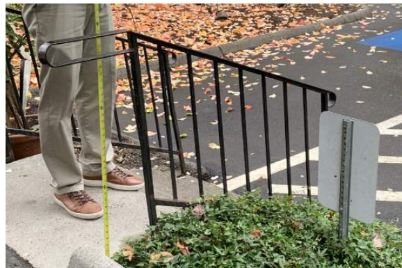
The handrail at the drive-through area is too low and not in compliance with code.
