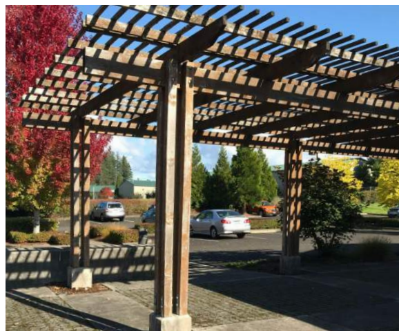
Wooden trellis is becoming covered in moss / lichen. It will likely need replacement / removal within the next 10 years.
