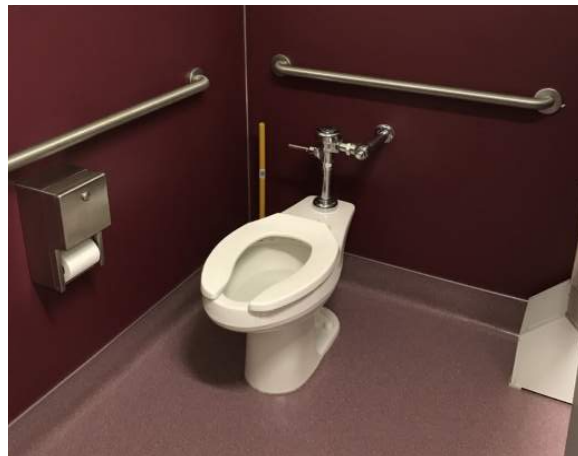
Restroom stalls in lower level do not meet ADA width requirements.
