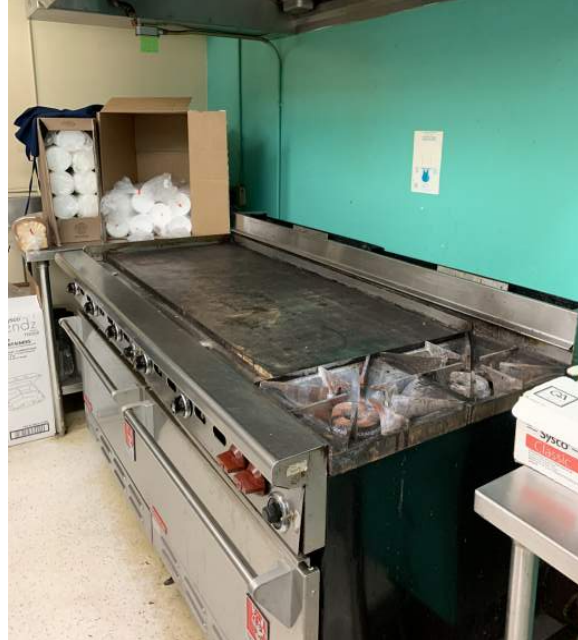
Equipment and flooring in the Community Center kitchen are in need of an upgrade.
