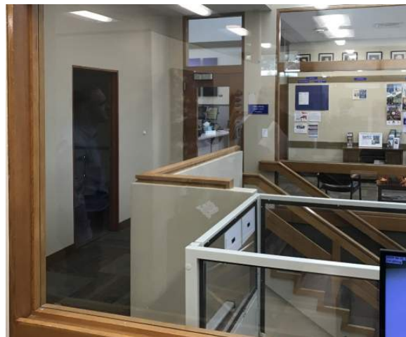
Potentially challenging ADA circulation in this area.
