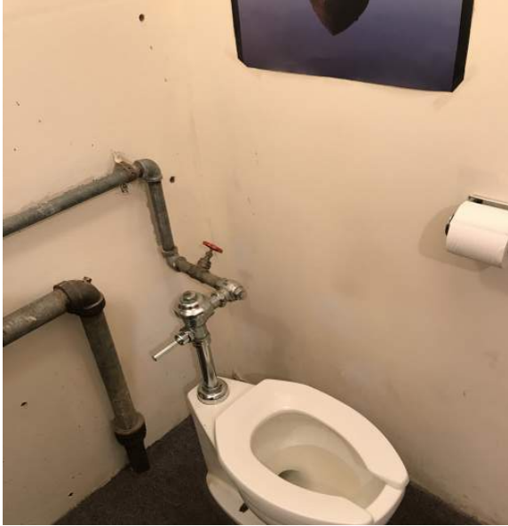
Non-ADA compliant staff restroom.
