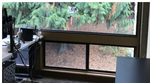
Low operable window in west facade is a potential safety hazard
