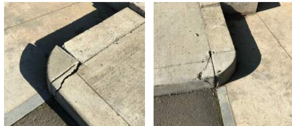
Damaged curbs around the bus wash station.
