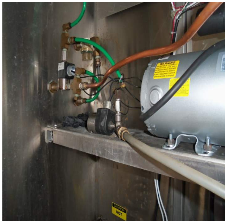
Vacuum Prime System Before
