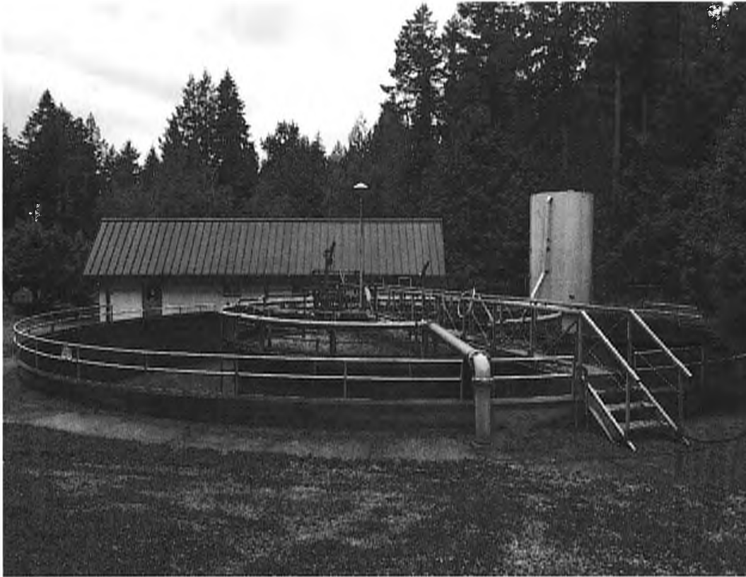
Aerated Sludge Storage Tank
