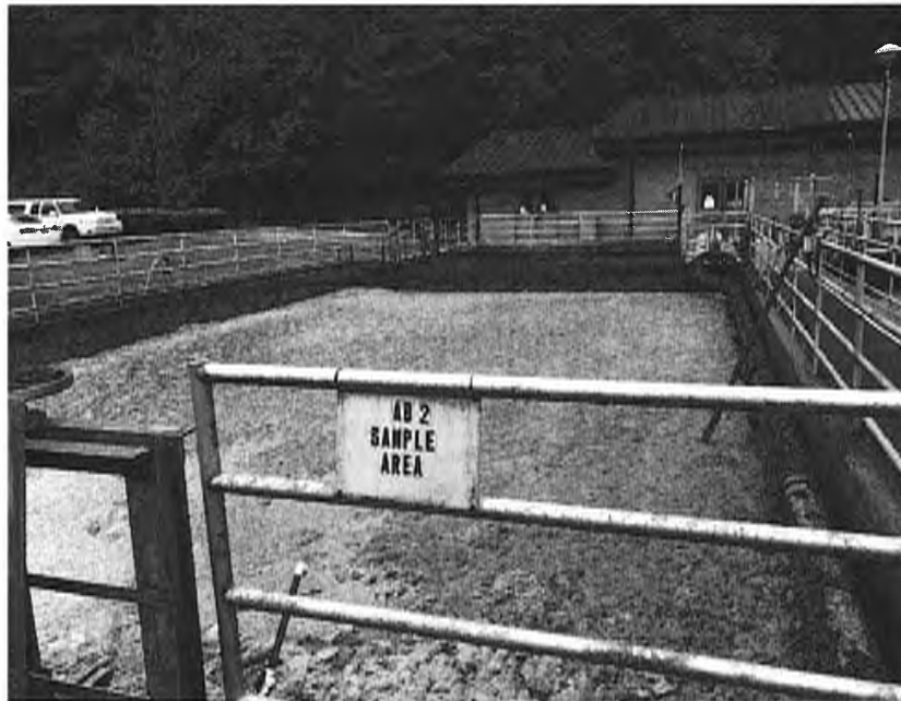
Aeration Basin No. 2 (Cell No. 8)
