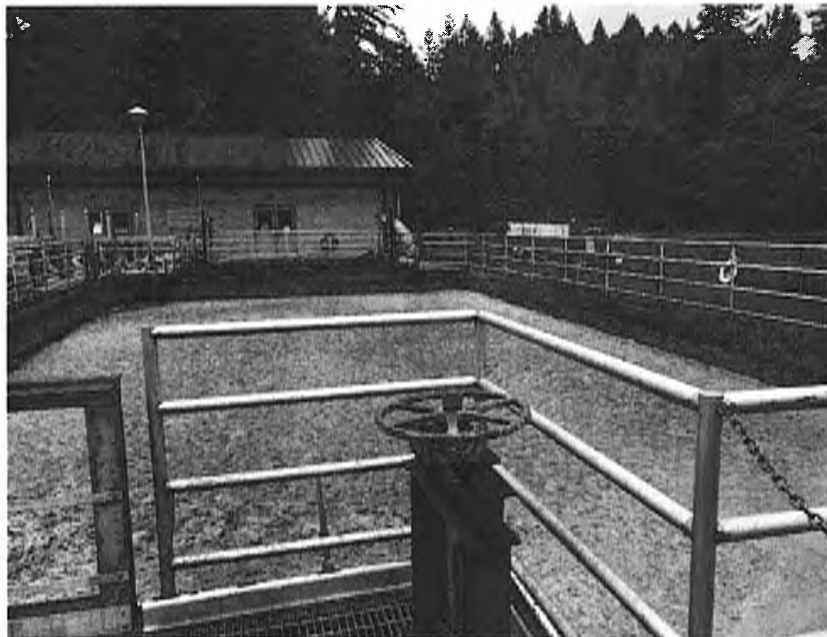
Aeration Basin No. 1 (Cell No. 4)
