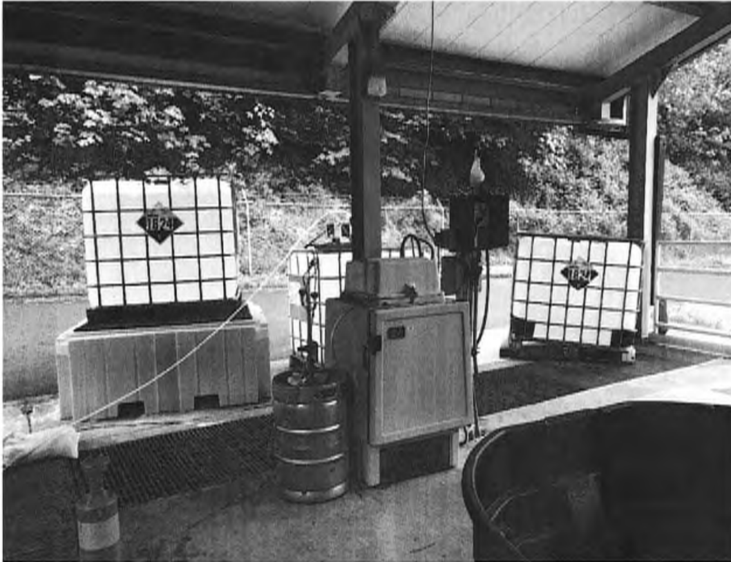
pH and Alkalinity Adjustment system at Headworks
