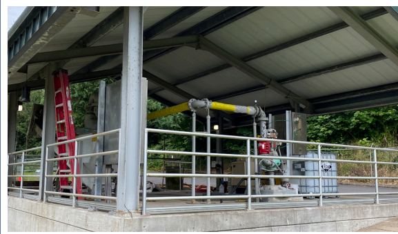
Figure 3. The existing 100 hp blowers appear to be in good operating condition.
