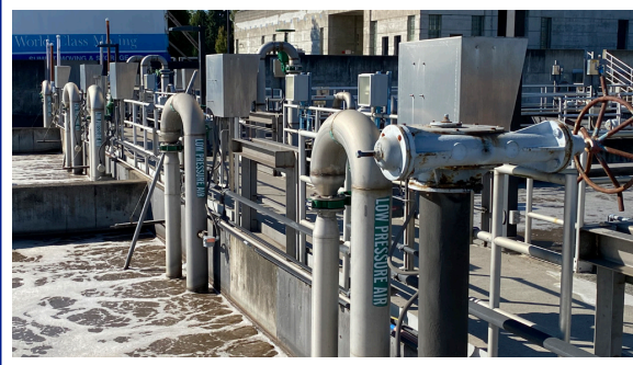
Figure 6. Installation of proper air drops with butterfly valves and air mass flow meters will improve aeration system performance and help protect blowers.
