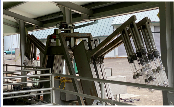
Figure 5. The existing UV system is still support by Trojan.
