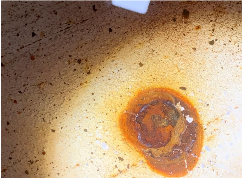
FIGURE 4 - TANK FLOOR PITTING
