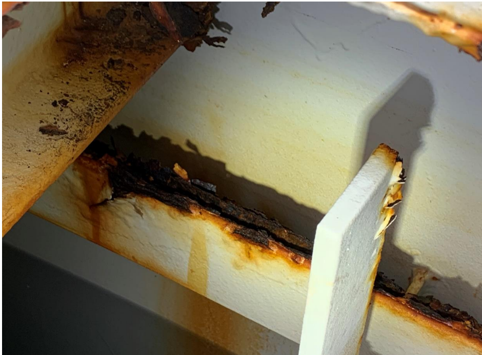
FIGURE 3 – DELAMINATION OF TANK STEEL AT ROOF ACCESS HATCH
