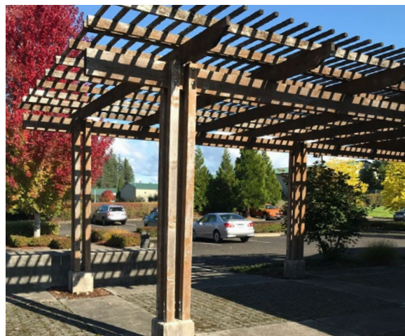
Wooden trellis is becoming covered in moss / lichen. It will likely need replacement / removal within the next 10 years.
