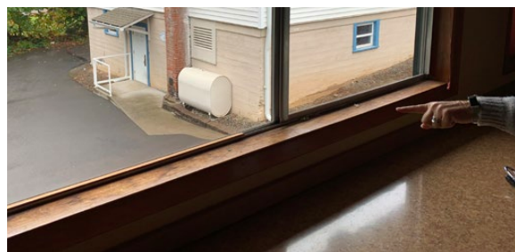
This operable window adjacent to a seating area in the Auditorium, 2 floors above grade, presents some safety concern amongst staff.
