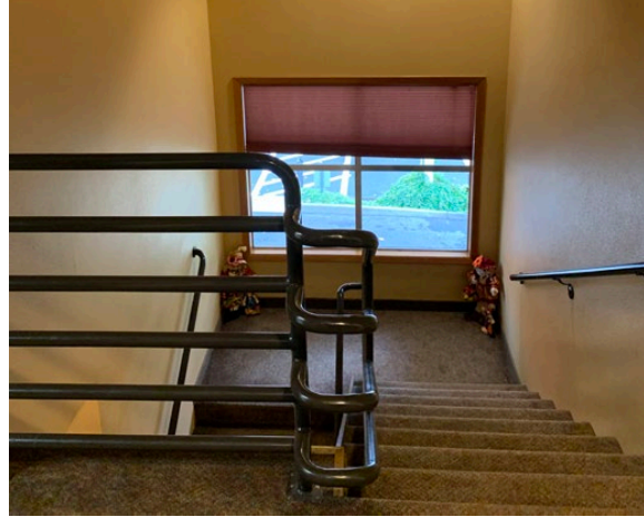
The main stairway at the Community Center does not provide a code compliant guardrail, and the window at the landing needs to be tempered safety glass in order to meet code as well.
