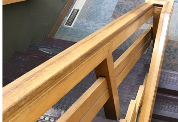
The wooden handrail is not in compliance with current code for handrail height, or width of the grip.
