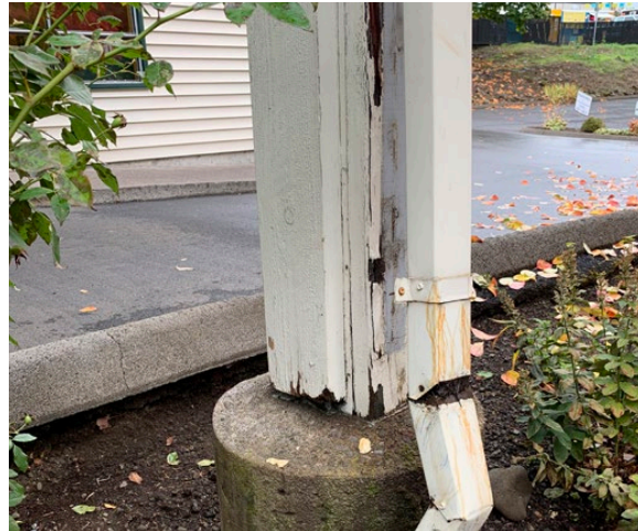
The main columns holding up the drive-through dropoff canopy are deteriorating and should be replaced or removed in the near future.
