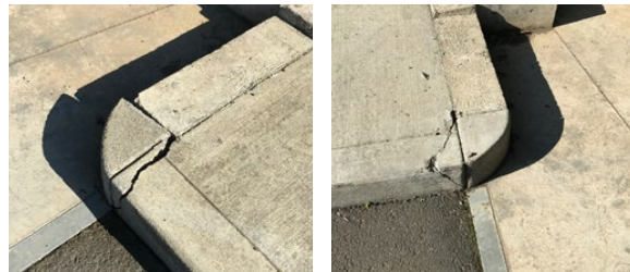
Damaged curbs around the bus wash station.
