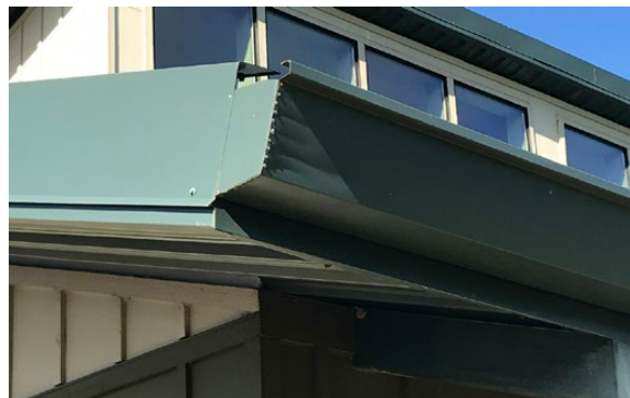
Several areas of gutter, such as this one, are in need of repair. Mechanical fasteners should not be used.
