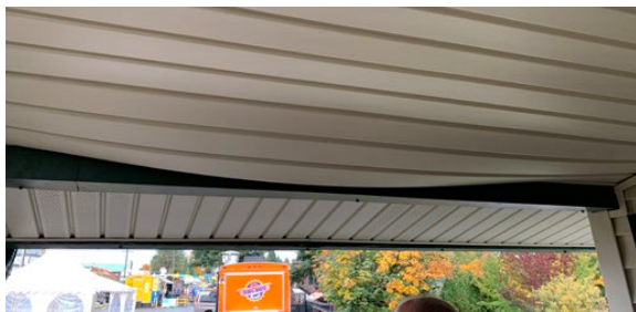
Vinyl soffit in disrepair at front porch.
