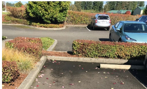
The formerly pervious paving in the front parking area now collects water and is not drained, creating flooded areas.
