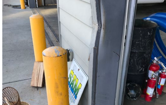
Damaged jamb at Public Works Building #3.
