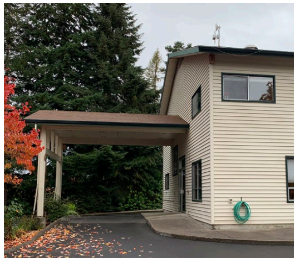
The drive-through dropoff entry is in need of structural repair or removal.
