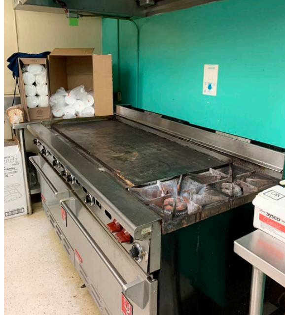
Equipment and flooring in the Community Center kitchen are in need of an upgrade.
