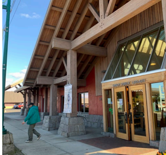
Wood elements at the Library entrance are likely to need refinishing and maintenance more often than other exterior elements.
