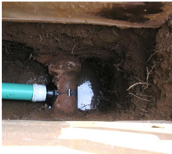
FIGURE 2. ADDRESSING LATERAL CONNECTIONS IS A KEY TO EFFECTIVE I/I REDUCTIONS
