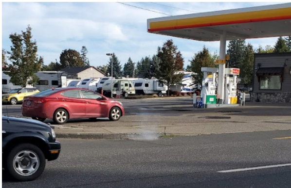
FIGURE 3. REMOVAL OF I/I IN BASINS 6 AND 7, SUCH AS THIS LEAKING CATCH BASIN, WILL REQUIRE CLOSE COORDINATION WITH OTHER STAKEHOLDERS, LIKE ODOT
