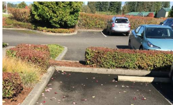
The formerly pervious paving in the front parking area now collects water and is not drained, creating flooded areas.
