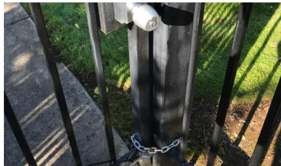
Gate entrance is chained due to people being able to reach through gate and open from inside.
