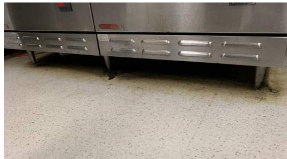
Linoleum flooring in the kitchen is beyond its life cycle and should be replaced.
