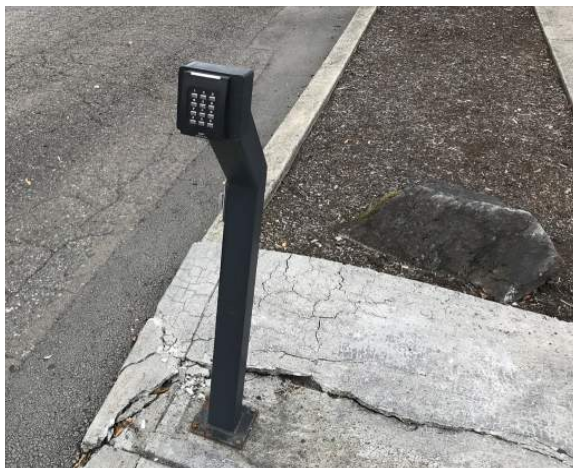
Damaged concrete driveway at secure parking entry area.
