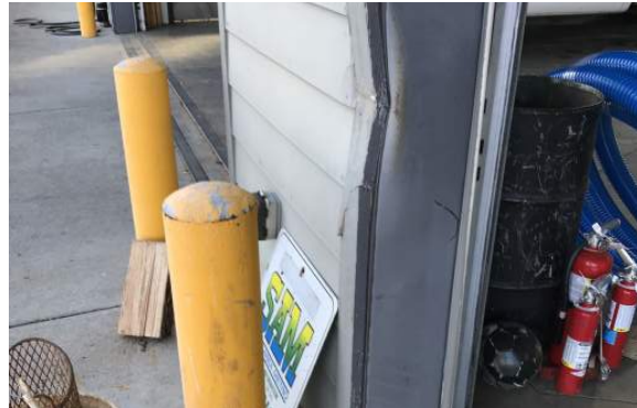
Damaged jamb at Public Works Building #3.
