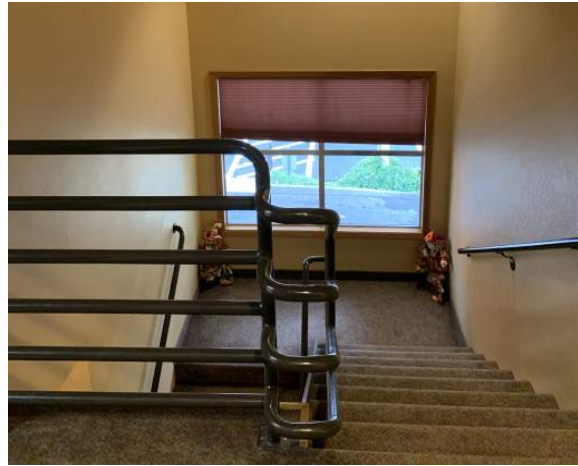
The main stairway at the Community Center does not provide a code compliant guardrail, and the window at the landing needs to be tempered safety glass in order to meet code as well.
