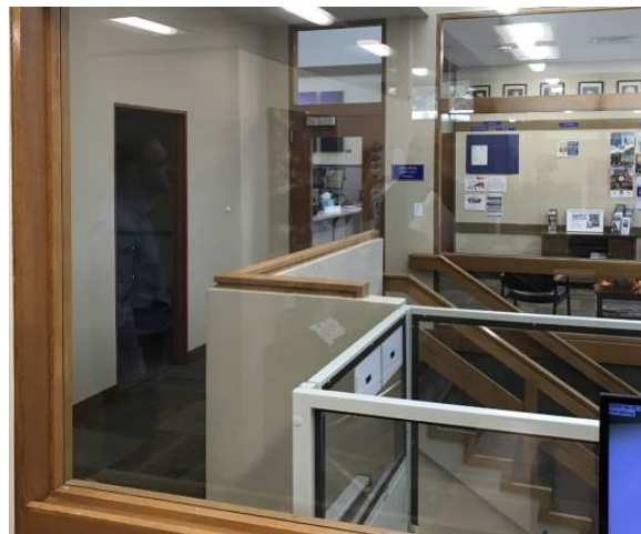
Potentially challenging ADA circulation in this area.
