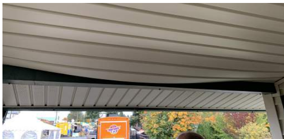
Vinyl soffit in disrepair at front porch.
