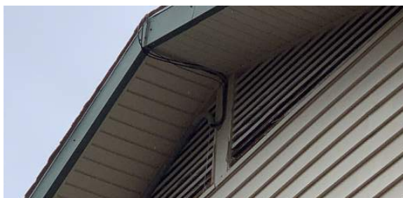
A vented area of the upper exterior wall appears damaged.
