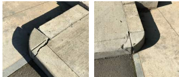
Damaged curbs around the bus wash station.
