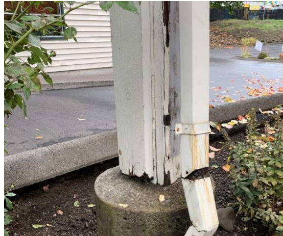
The main columns holding up the drive-through dropoff canopy are deteriorating and should be replaced or removed in the near future.
