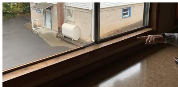
This operable window adjacent to a seating area in the Auditorium, 2 floors above grade, presents some safety concern amongst staff.
