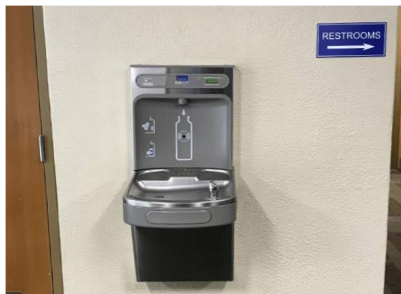
Single-height drinking fountain in lower hallway needs to be dual-height to meet ADA criteria.
