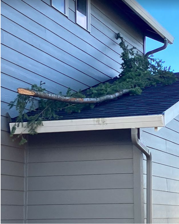
Image 5: Failed branch on client's house
