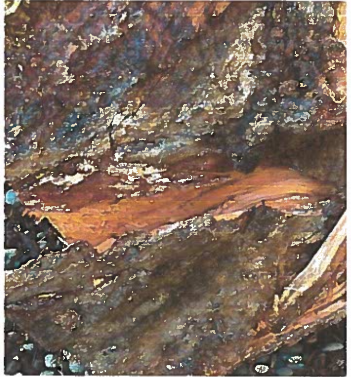
Image 5: Evidence of Doug-fir beetle and decay
